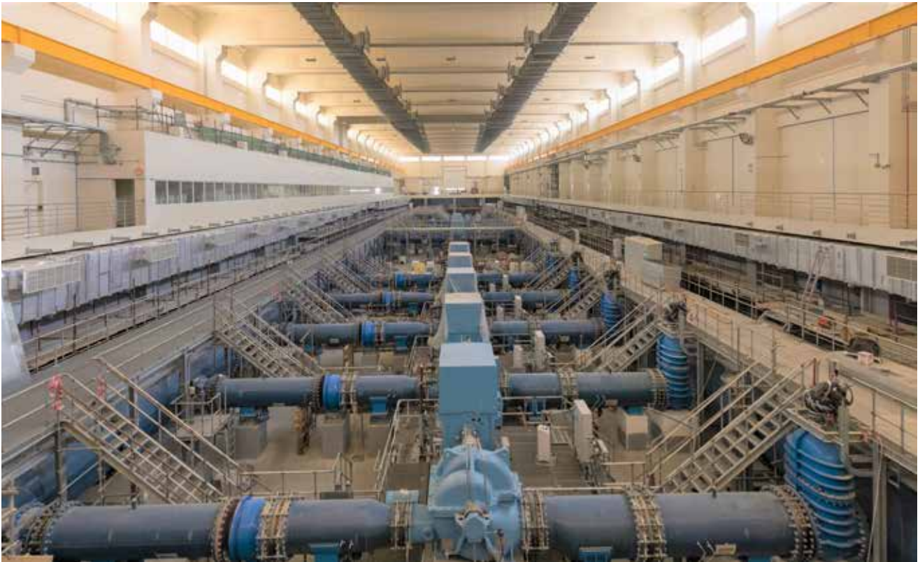
Main Pumping Station of PRPS 4 – Abu Nakhla © Tractebel GWK
